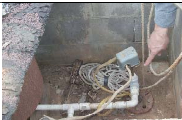
Figure 1. Example of poorly constructed well, flush to the ground, allowing surface water to enter the casing.
